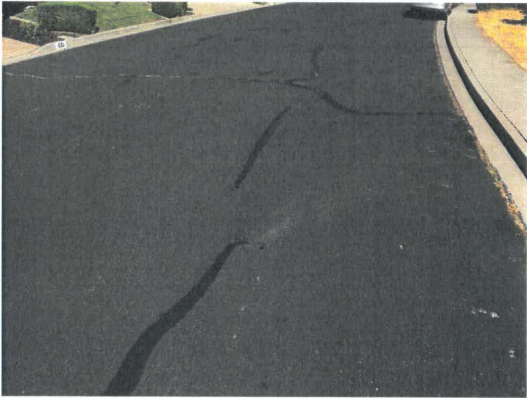
PHOTO 1 - 2016 CRACKS IN PAVEMENT, PEBBLE BEACH DRIVE
