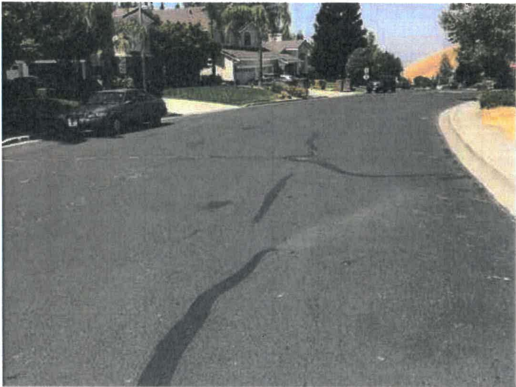
PHOTO 2 - 2017 CRACKS IN PAVEMENT, PEBBLE BEACH DRIVE
