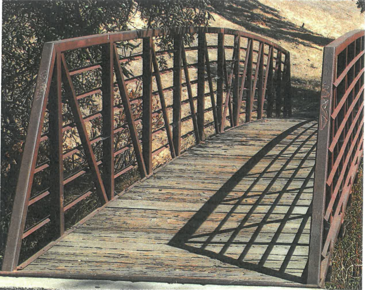
Before – decay wood
